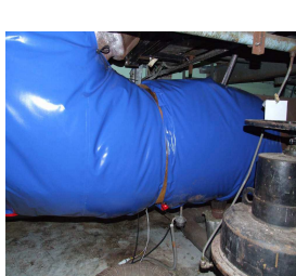
Huge industrial pipe
